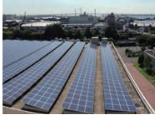
Photovoltaic power generation using the upper space of a sewage treatment facility (Kanagawa Water Reclamation Center)
