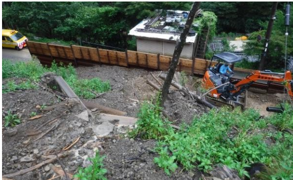
Landslides caused by heavy rain (July 2023)
