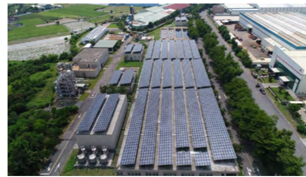
Installation of Solar Energy Equipment on Industrial Park Factory Roofs in Kaohsiung City
