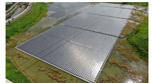
Floating PV Technology at Wujiawei Water Detention Basin
