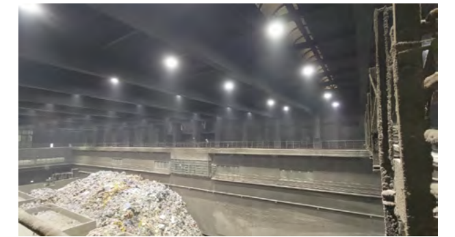
Replacement of Old Lighting Fixtures with High-Efficiency LED Fixtures at Gangshan Incinerator Bunker Area
