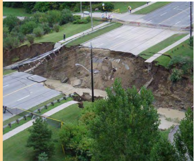
DAMAGE FROM AUGUST 19, 2005 STORM (PHOTO FROM JANE-FINCH.COM)
