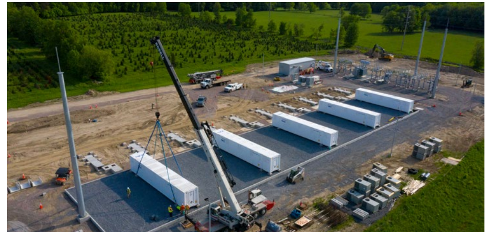
Construction of new battery storage facility, adjacent to Willis Substation, part of NYPA's St. Lawrence-FDR Power Project.
