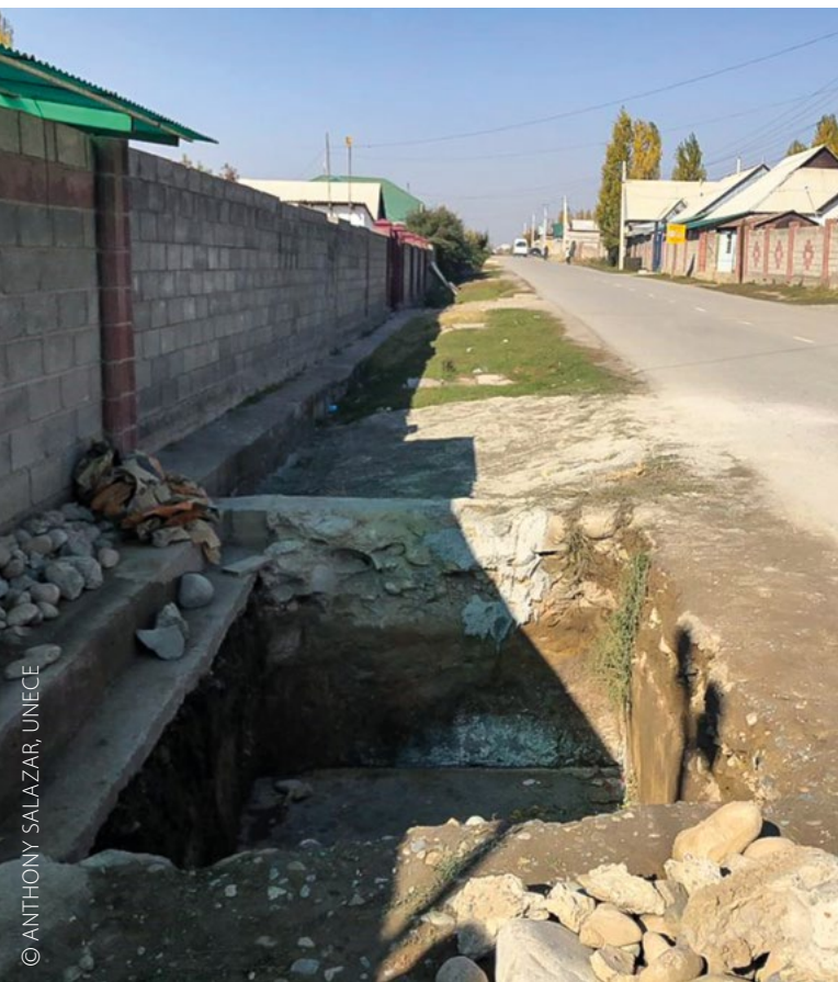
Individually constructed septic tank, Kalis Ordo informal settlement
