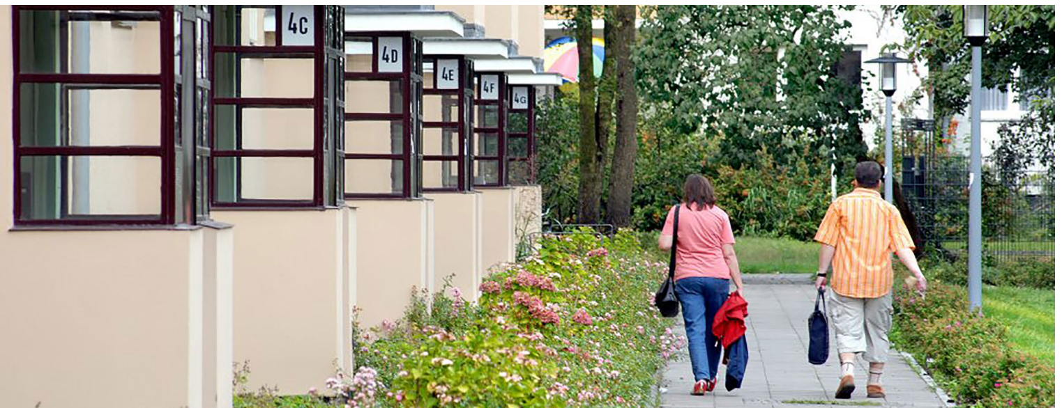
Renovated windscreens on residential buildings in the settlement Haselhorst enable less heat loss
