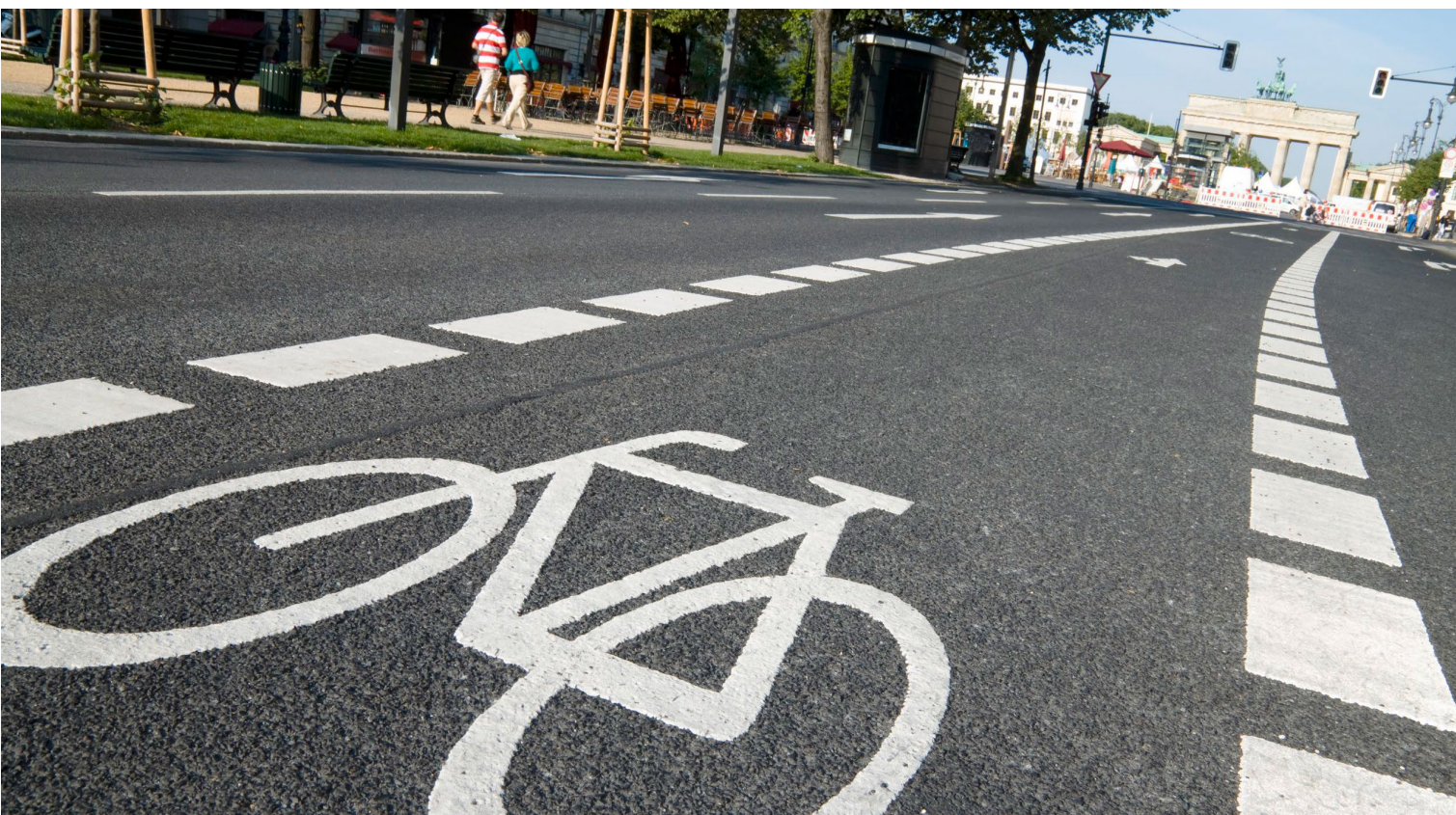
More routes by bicycle: The final report for a BEK suggests expanding the cycling infrastructure
