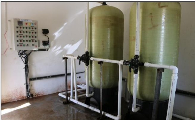
Image : STP plant at Bopal Garden
